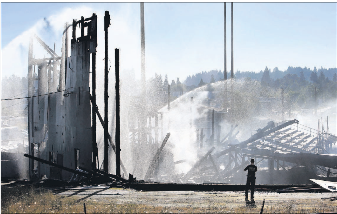
A firefighter takes a photo of the smoldering remains of Civic Stadium, June 30, in Eugene.
