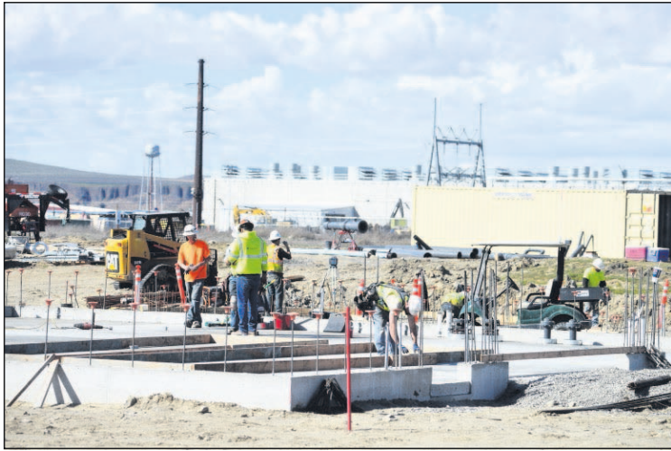
Staff photo by E.J. Harris A construction crew works on a water treatment facility that will serve data centers at the Port of Umatilla on Wednesday in Umatilla.
