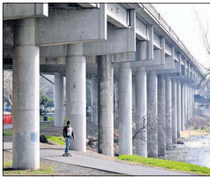
This Feb. 13, 2013, file photo, shows the viaduct that carries Interstate 5 traffic for more than a half mile over Bear Creek and city streets in Medford.
