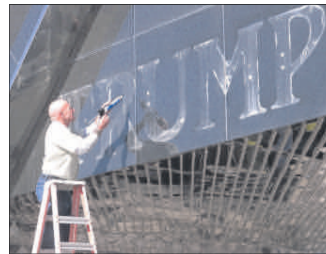
In this Oct. 6 photo, a worker applies caulk to holes in the facade of the former Trump Plaza casino in Atlantic City N.J. after letters spelling out the casino's name were removed. The casino closed on Sept. 16.
