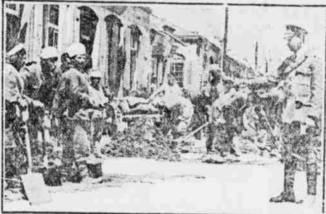
Besides feeding the Armenians, the Near East relief workers are teaching them the value of good roads by building them. Workers are paid in food. Photo shows Clifford Downer of Kingston, N. Y., directing a road gang at Alexandropol.
