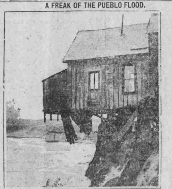
A freak of the Pueblo flood. The kitchen of this house is hanging over the embankment without any support, except the long beams that reach out from the part of the — see left on land.
