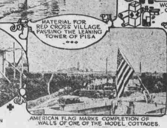
AMERICAN FLAG MARKS COMPLETION OF WALLS OF ONE OF THE MODEL COTTAGES.
