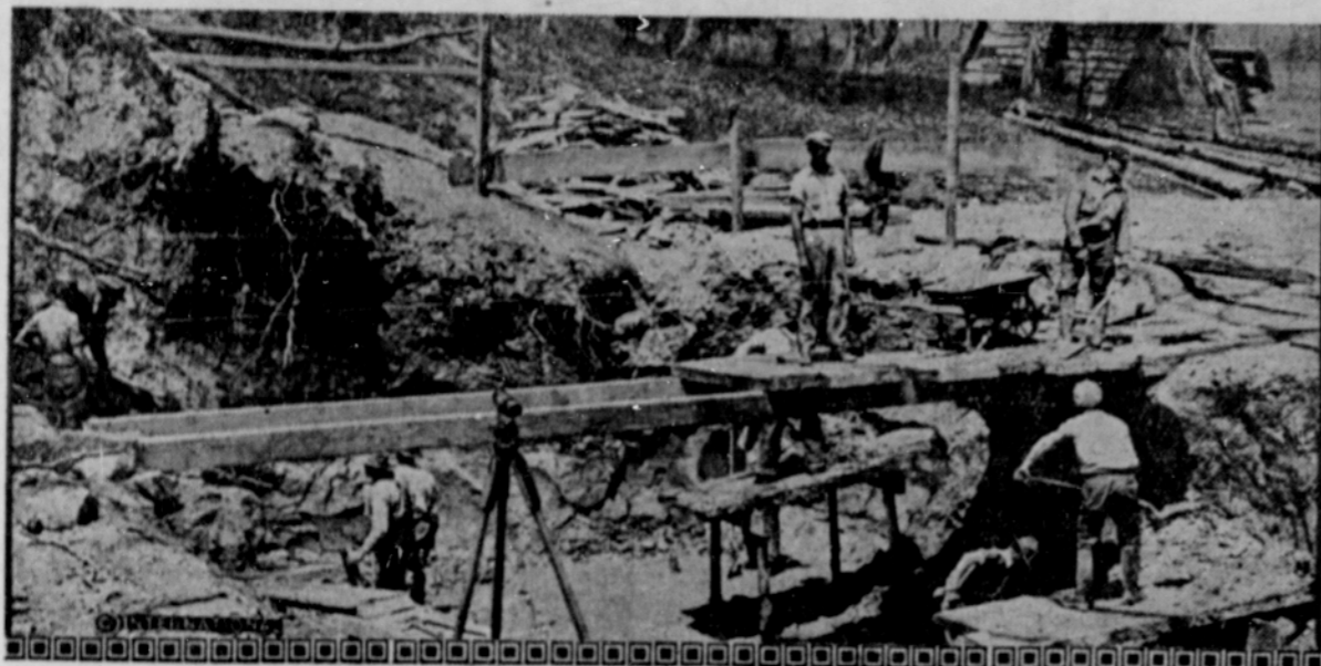
Liquors, whisky and brandy were made for home consumption at George Washington's still house near his mansion at Mt. Vernon. Workmen are shown repairing the historic structure as well as the old mill, some of the timbers of which have been unearthed and can be seen quite plainly.
