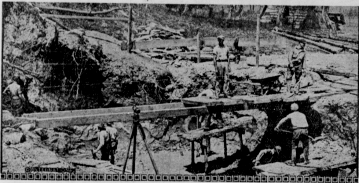
Liquors, whisky and brandy were made for home consumption at George Washington's still house near his mansion at Mt. Vernon. Workmen are shown repairing the historic structure as well as the old mill, some of the timbers of which have been unearthed and can be seen quite plainly.
