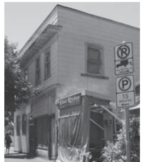
The Sons of Haiti Masonic Lodge – threatened with closure due to building code issues and fines – will stay open after a community fundraiser and assistance from the PDC.
