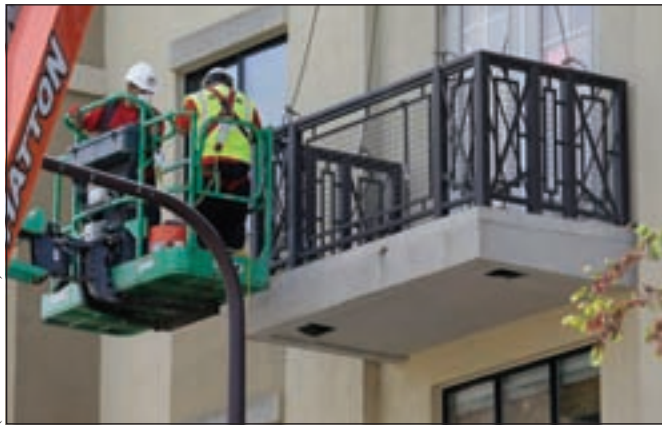
A crew begins work on the Library Gardens apartment building balcony below the remaining wood from a balcony that collapsed in Berkeley, Calif., Wednesday, June 17, 2015. The balcony broke loose from the building during a 21st birthday party early Tuesday, killing several people and seriously injuring others.
