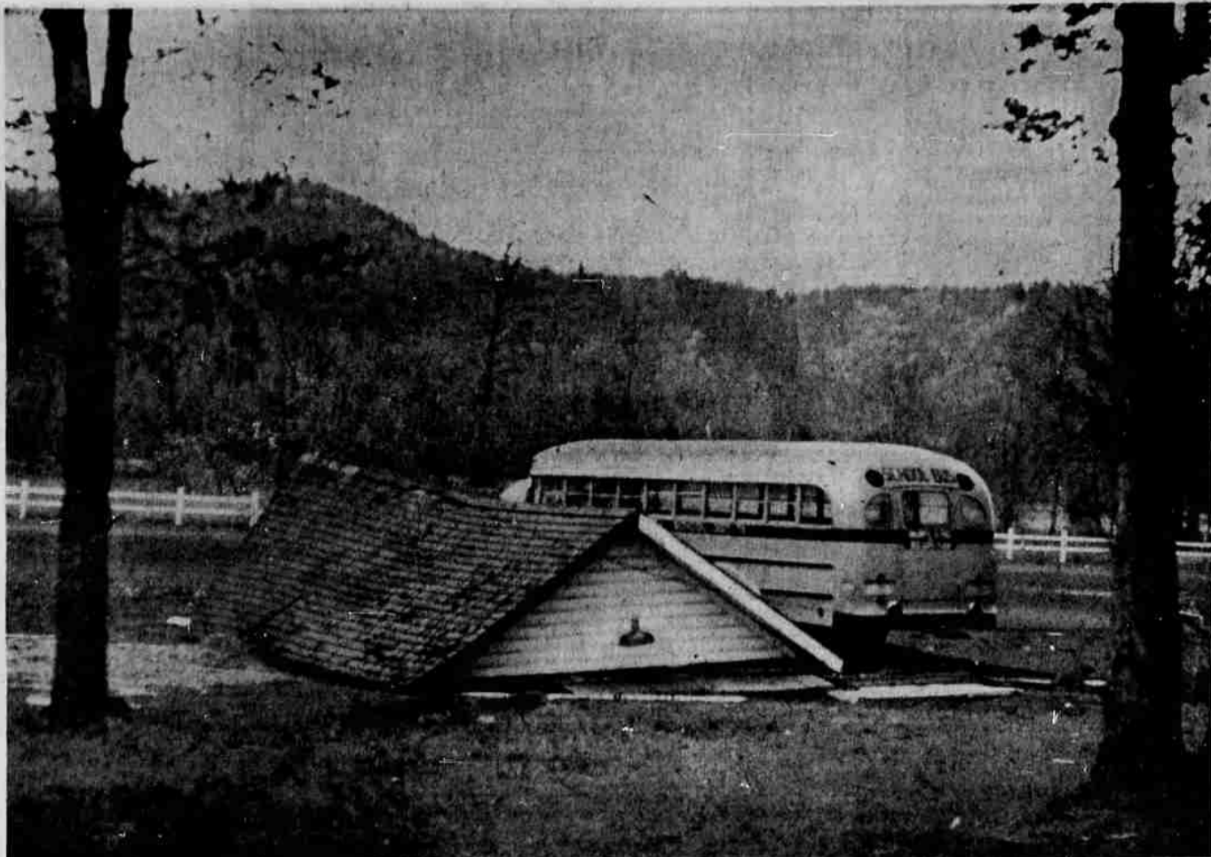
This Marcola school bus received only a dented hood when a wind gust hit the garage where it was parked. The roof was lifted into the air and came down on the collapsed walls of the garage. Some 20 houses in the Marcola area were damaged by falling trees.
