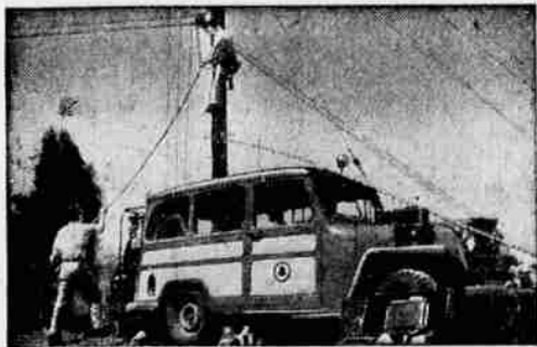
Radio trucks are spotted in many locations through the West to "bridge" breaks in wire lines. Emergency materials, too, are stockpiled in many places.
