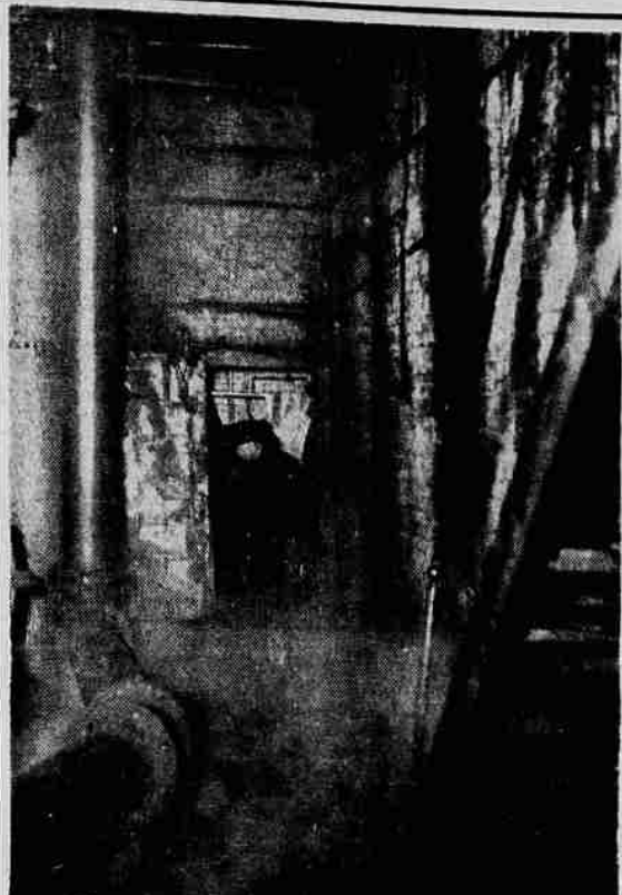
FIREMEN CHECK the Northwest Cities Gas Co. plant at the foot of Eighth Ave. for damage after an unexplained explosion, followed by fire, damaged the plant Friday evening. (Willshire photo and engraving.)
