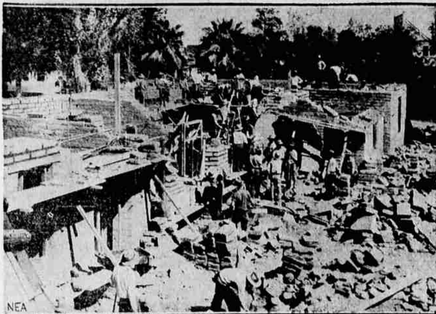
When Brawley, Cal., needed a new city hall and had only $4000 in cash, the mayor called in the citizens and a new adobe city hall, valued at $50,000, was the result. Citizens worked out delinquent taxes or took scrip, which was exchanged for groceries, and merchants in turn paid off taxes. Photo shows activity during construction.
