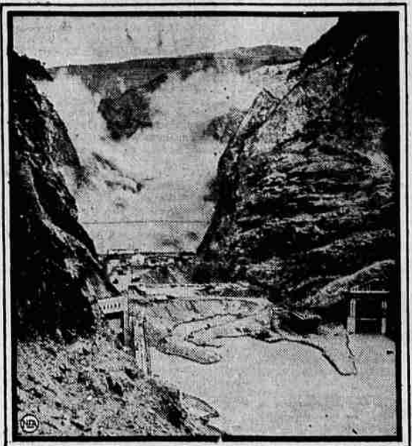
Four tons of dynamite blasted away a mountain of dirt and rock, marking the last "big shot" before actual construction of Hoover dam begins. The picture was taken as thousands of tons of rock fell into the Colorado river canyon. In the foreground may be seen the tunnel through which the river's flow has been diverted.
