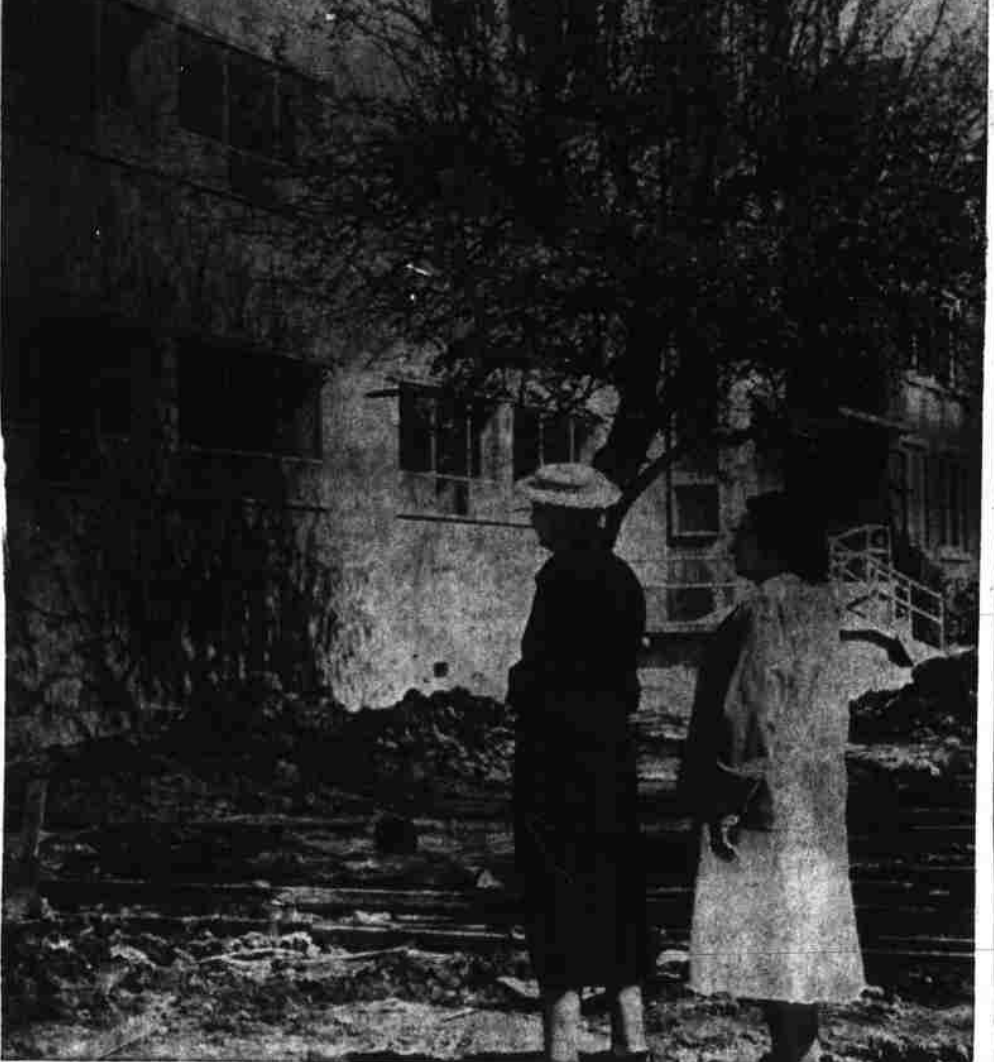
First two floors of the new wing at the Methodist Home, 1625 Center St. NE, are almost completed and will provide 21 new rooms. Looking over the project are Mrs. A. C. Poole (left), resident of the home, and Ruby Justis, a staff member. (Statesman Photo.)
