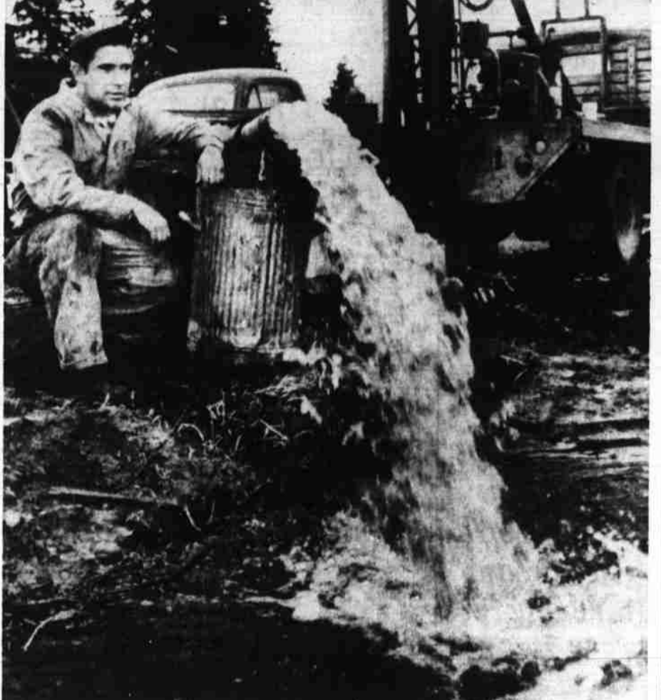
SALEM HEIGHTS, March 20—Newest well supplying Salem Heights Water District, located a half mile east of Liberty School south of Salem will supply a minimum of 1400 gallons per minute. Pumping Operator Eddie Hart happily watches discharge during test pumping this morning. (Statesman Photo)
