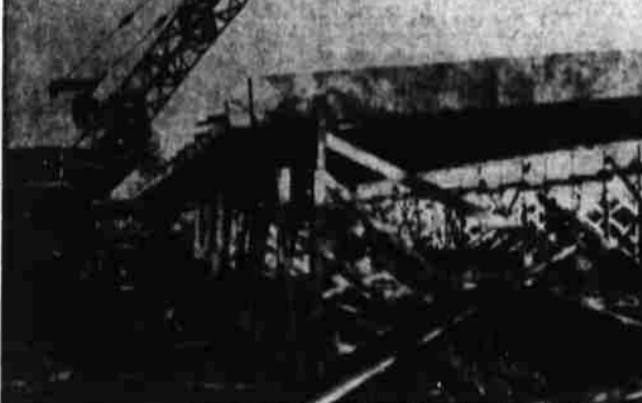
DALLAS, Jan. 12—Contractor John Steinmuller, Eugene, is pushing forward construction of new 8-classroom Whitworth Elementary School here despite bad weather. Laminated beams on classroom wing of building are shown being placed by big crane. The $265,000 building is expected to be completed by late spring to relieve crowded grade schools. Sea of mud surrounds present construction scene.
