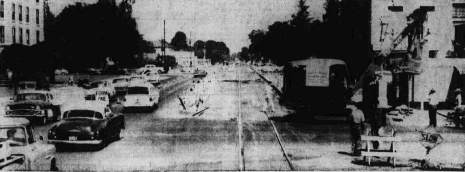
This photograph looking north from the intersection of 12th and State streets shows work progressing on 12th Street ravamping project. Elsewhere, work under a $250,000 city street improvement program is coming along on schedule. This summer's street program is one of the city's largest.
