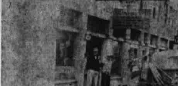
Unwelcomed shower on a hot day plasters C. M. Will, city water department crewman, as he contemplates a broken main Friday afternoon on South 12th Street. Spectacular spray shot 40 feet into the air as a fitting on a 4-inch main broke while workmen were attempting to repair a damaged pipe. Break occurred just south of Mill Street, where 12th Street widening project is going on.
