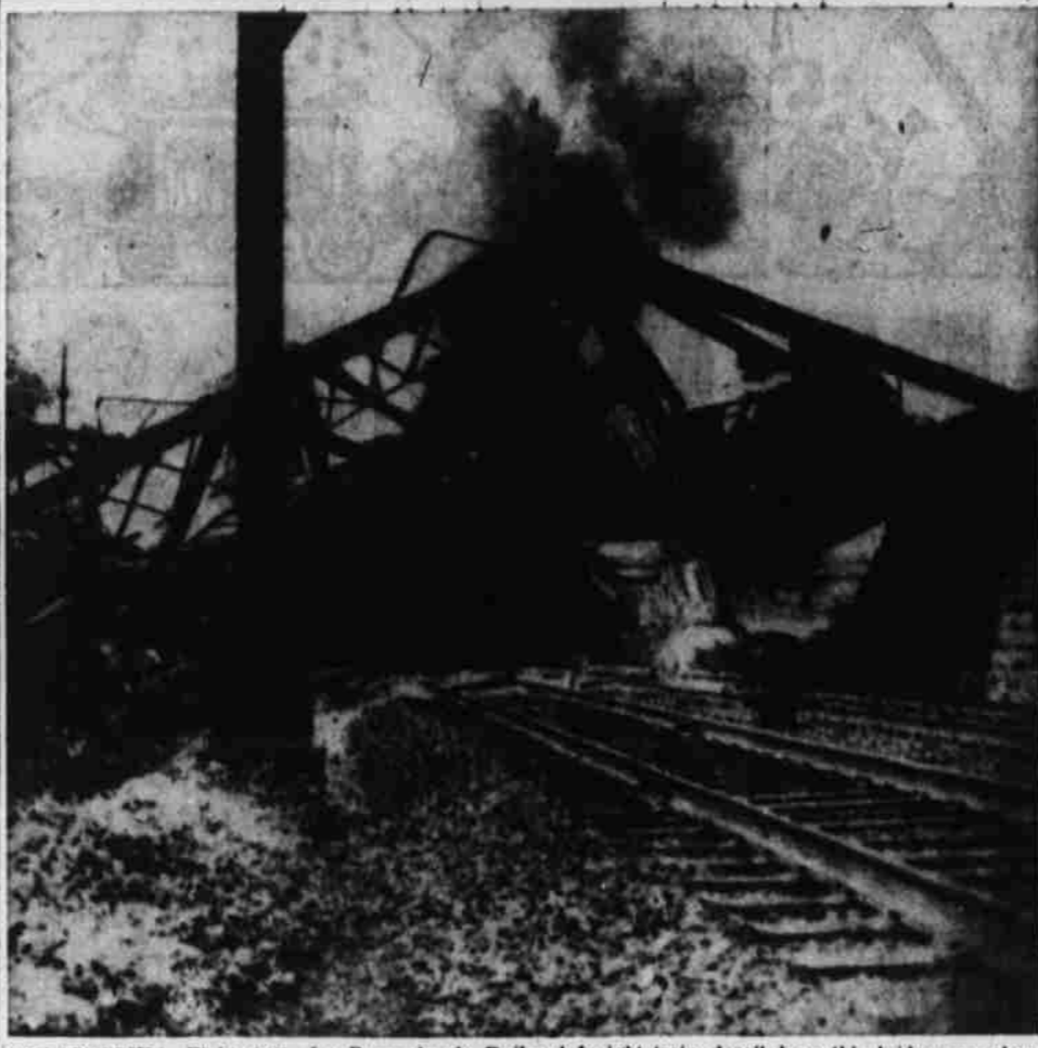
PHILADELPHIA—Eight cars of a Pennsylvania Railroad freight train derailed on this bridge near here Saturday, collapsing the bridge and plunging to tracks of the Reading Co. below. Both lines were blocked. Some of the wreckage caught fire. There were no casualties. (AP Wirephoto.)
