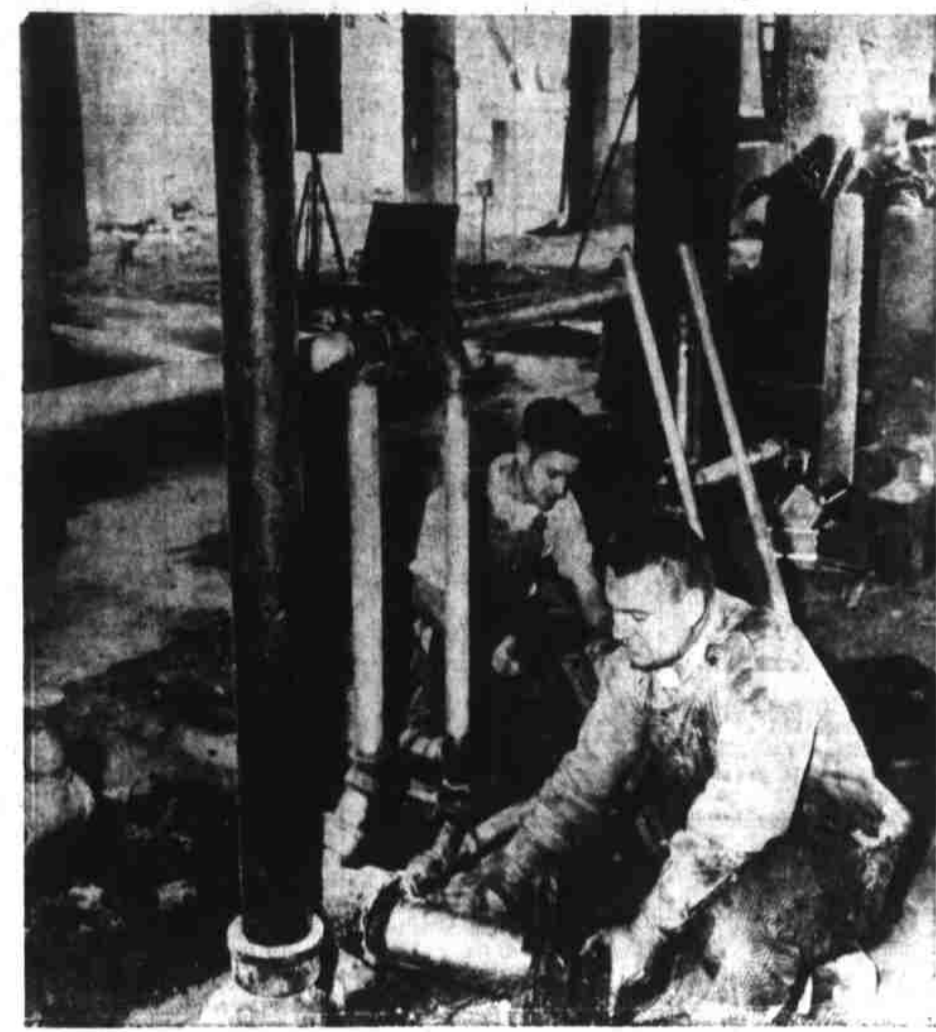
Plumbers Harold Ewart (in rear) and R. G. Zimmerman work on pipes in basement of the new wing of Salem YMCA. Work on the structure is progressing rapidly and is expected to be completed in early October. Pipes shown here will furnish water for men's shower room. (Statesman Photo).
