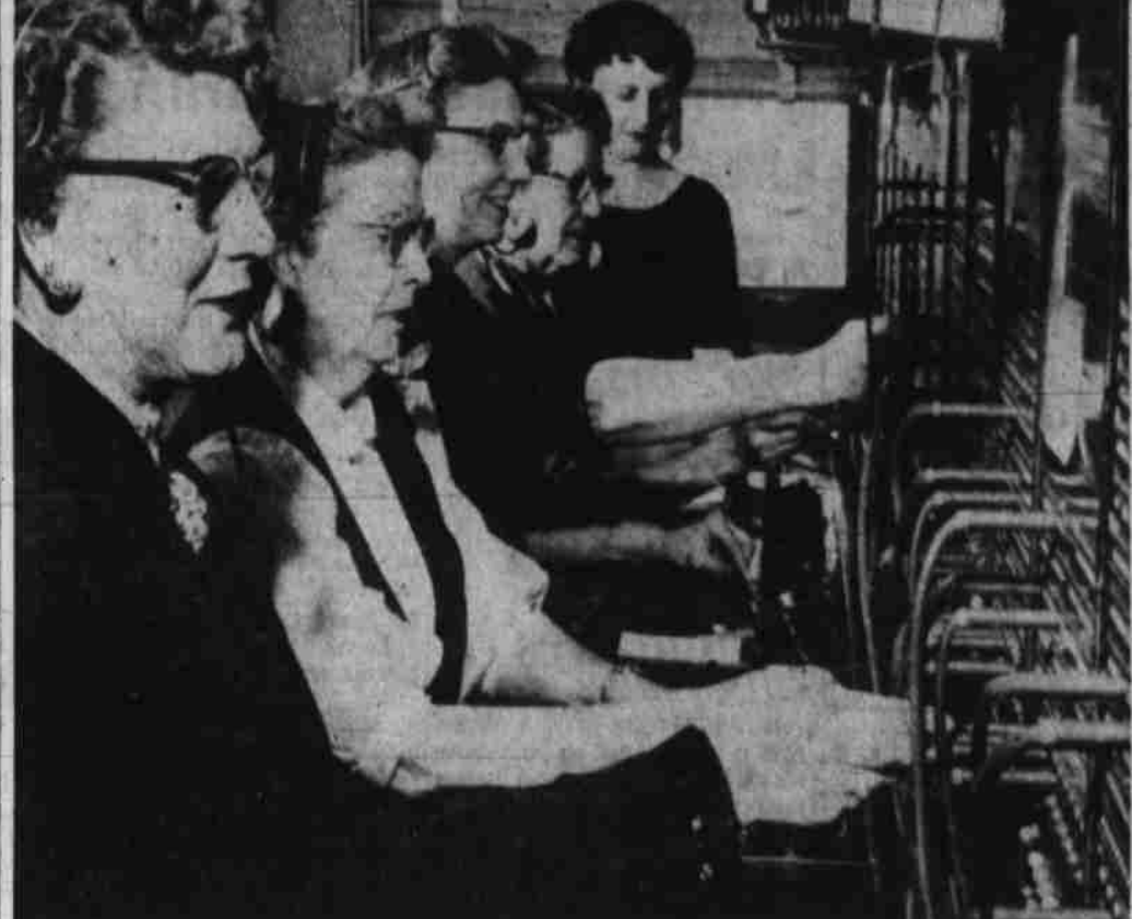
One of the busiest telephone switchboards in Oregon is the board at the state capitol in Salem (shown above) which handles the daily flood of incoming calls for hundreds of state officers. Operators shown at work at the board located in the old state office building are (from left) Jennie Madison, Cleo Surprenant, Peg Ritchie, Peral Pack and their supervisor Mrs. Irene Cross. Swinging files above their heads holds names and extension numbers of some 4,800 state employees. (Statesman photo.)
