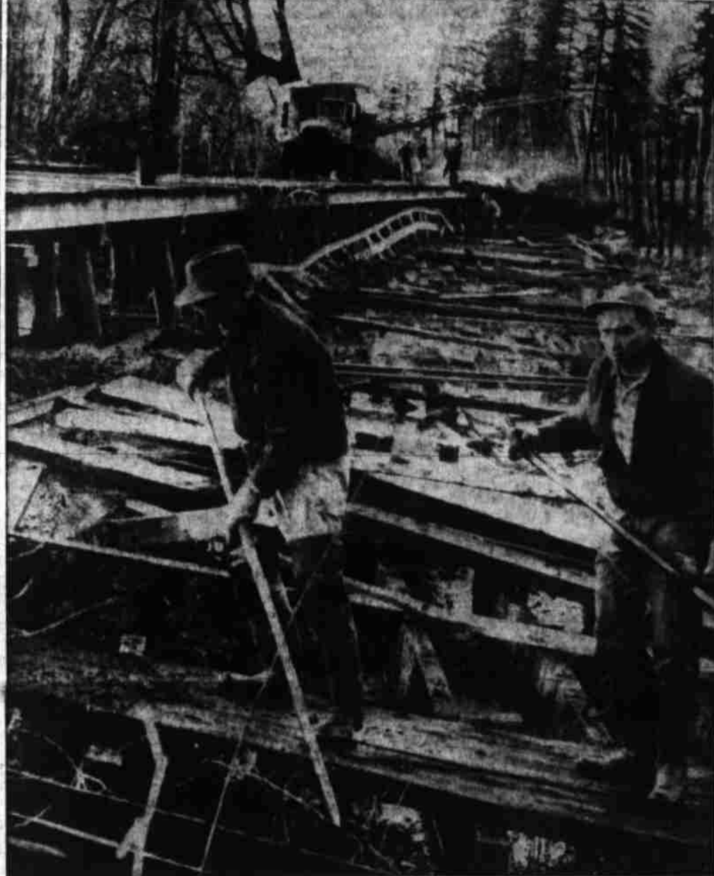
Marion County bridge crewmen are shown Tuesday shortly after noon rebuilding a flood-damaged bridge in the Mission Bottom area north of Salem. Two crewmen, Virgil Fahey, left, and Bob Martin, are shown in foreground salvaging planking from wrecked span's deck to be placed back on original undamaged pilings (at left). When bridge was opened marooned families streamed over. (Statesman photo).
