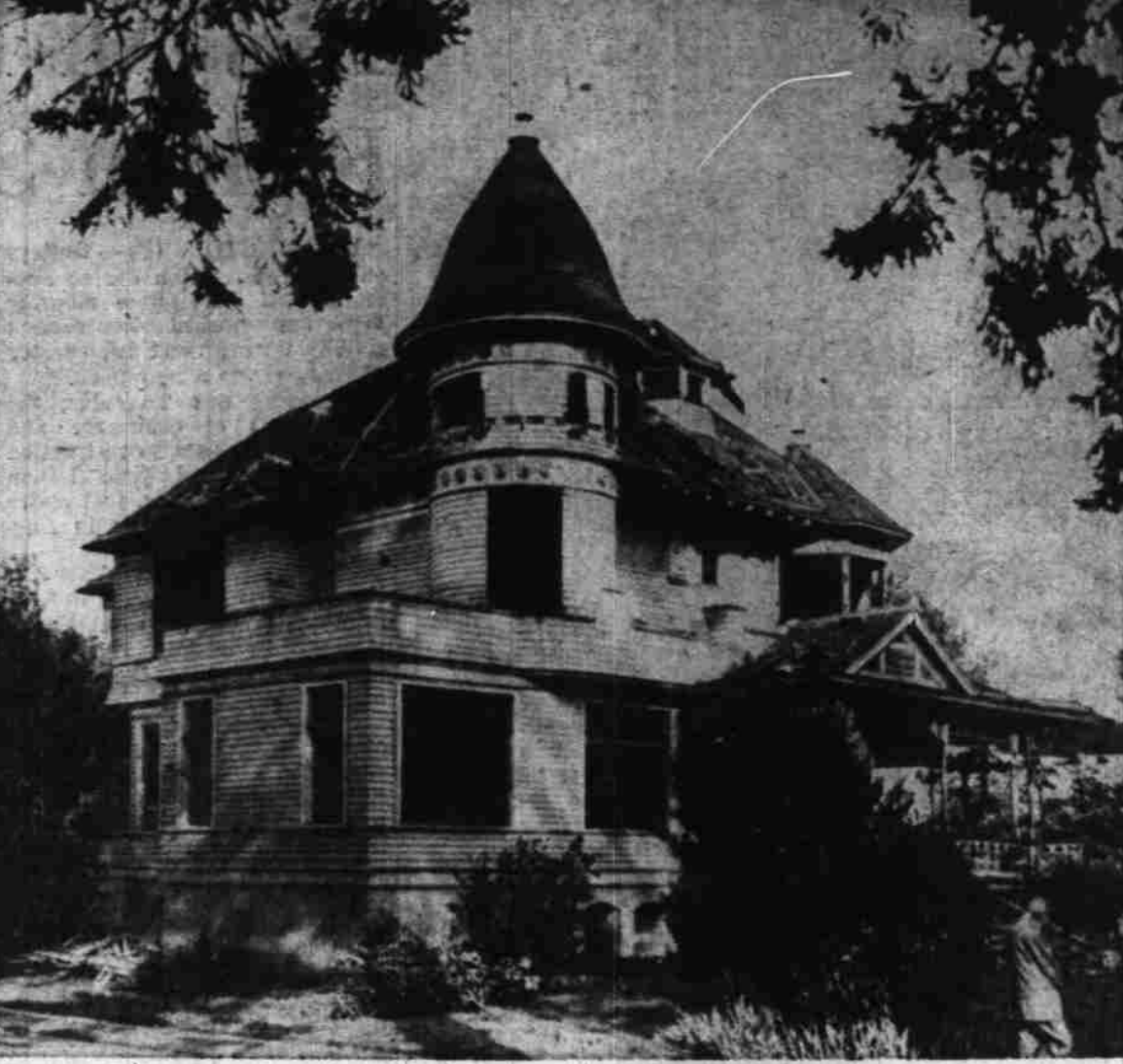
Residential landmark between downtown and the Capitol is this C. P. Bishop house, an elegant home of Salem's yesterday which now is being torn down. The Court Street property has been acquired by First Presbyterian Church.
