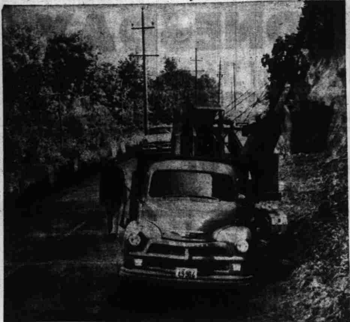
Digging work by one of Jake Wright's city engineering department crews was completed Tuesday on first phase of the newest South River Road improvement—a $22,000 city project extending about one-half mile from Miller Street to city limits. Here the paved surface will be widened from 16 to 26 feet, a 4 1/2-foot sidewalk will be placed on the east side and curbs on both sides. Curbing work will begin next week, following a plan designed to keep half the roadway open to traffic. (Statesman Photo.)
