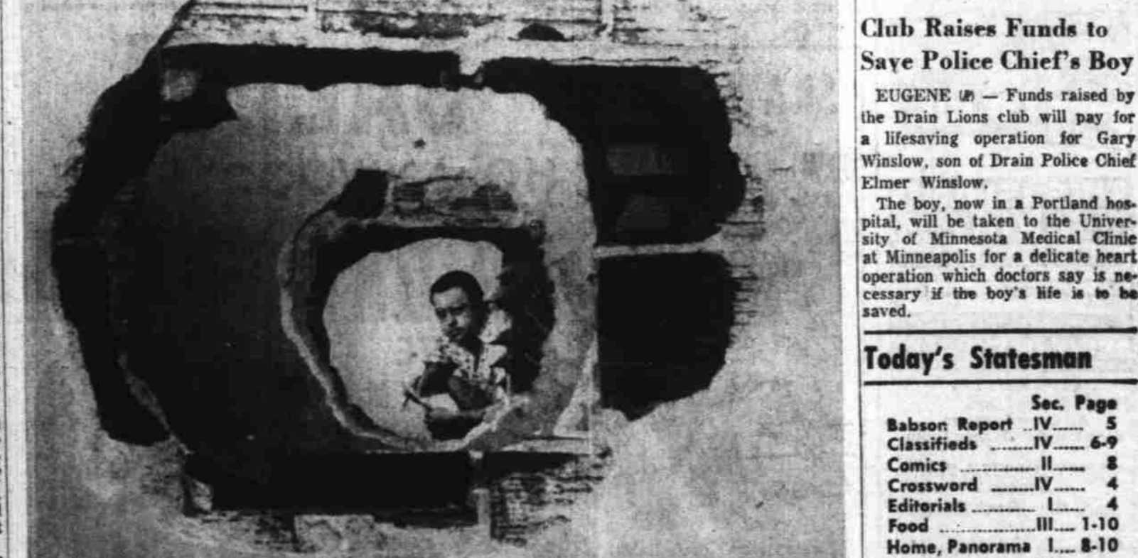
Although most of the debris had been cleaned up Thursday these big holes in room walls remained as evidence of the destructive violence Wednesday night at the State's Hillcrest School for Girls near Salem. Above is shown Statesman reporter Conrad Prange peering through a row of holes pounded through the plaster-hollow tile walls by girl inmates of the maximum security unit. (Statesman Photo.)
