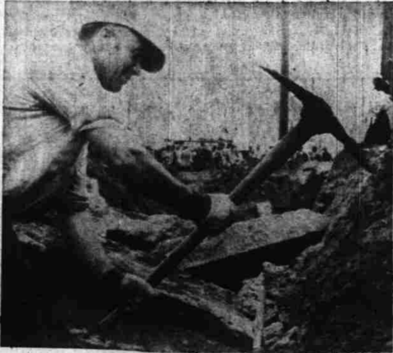
While costumed girls and business-suited insurance men and city leaders did the formalities of groundbreaking for Allstate Insurance Co. office building in downtown Salem Wednesday noon, workman Clarence Mackintosh swung his pick in some of the actual excavating work beneath level of Ferry St. (Statesman Photo.)
