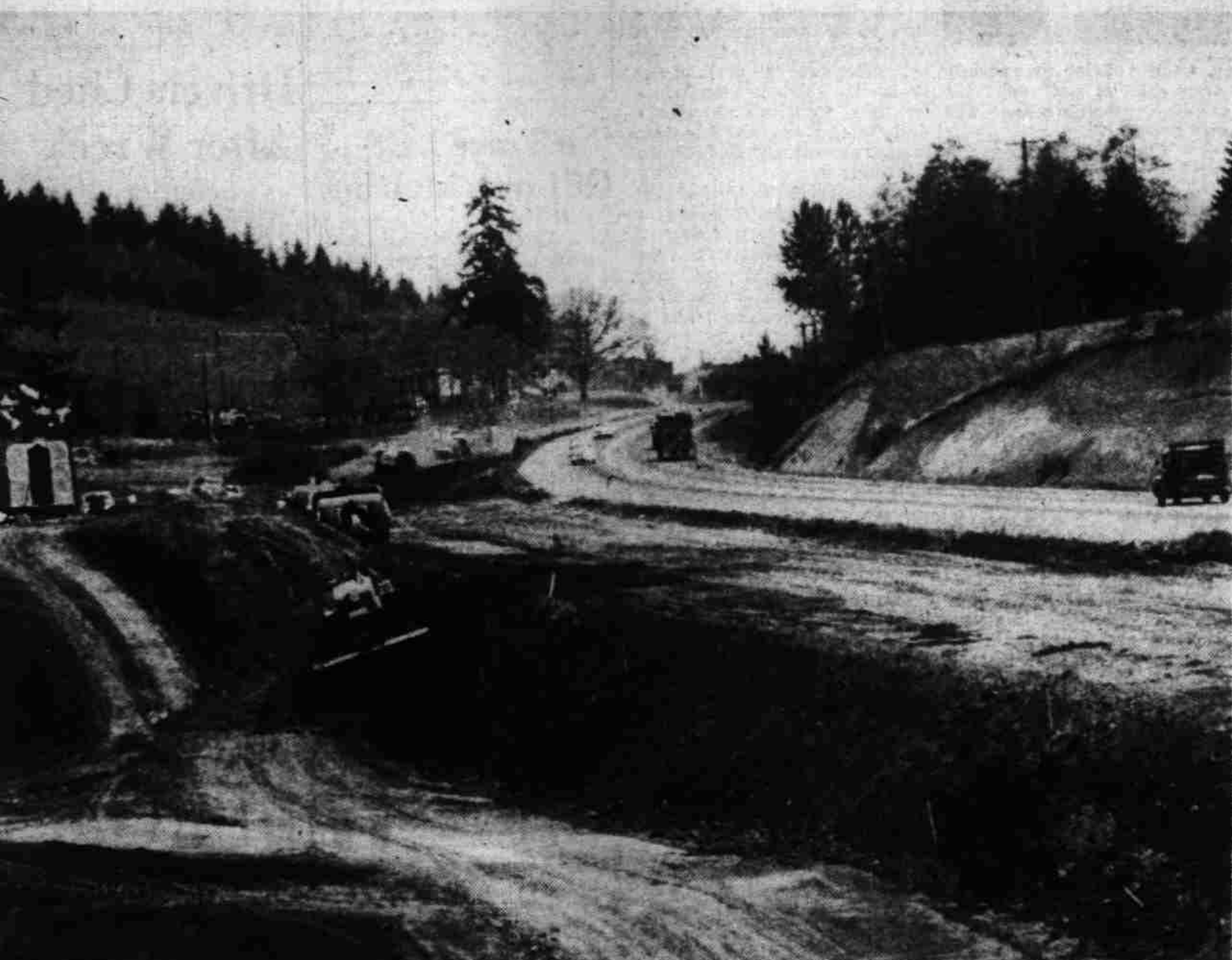
Bulldozers and other equipment are shown at work here on a new section of Highway 99E south of Salem. The site is just south of Illahee Hill and the camera is facing north. When completed the work going on in the foreground will provide two additional one-way lanes to become a part of the present highway (in background) which will also carry two lanes one-way, according to state highway department officials. When completed, probably early next year, the new one and one-half mile section will be the first link in a proposed four-lane expressway from Salem to Albany. The Salem-Portland section is practically completed. (Statesman photo.)
