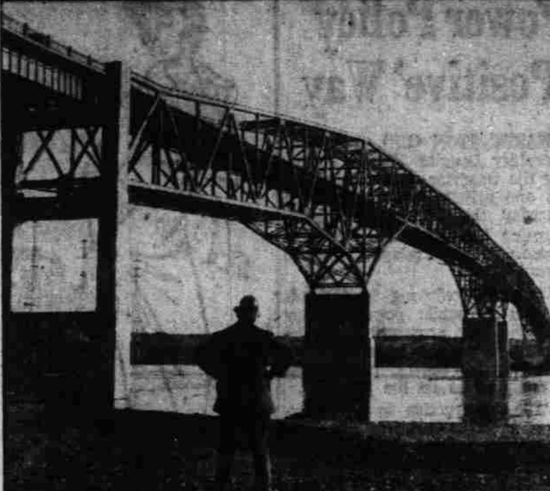
UMATILLA, Ore. — Traffic time-saver nearing completion in the Northwest is this new span being built by U.S. Steel's American Bridge Division across the Columbia River at Umatilla, Ore., just below McNary Dam. The 3500-ton steel crossing will replace a ferry operated by Umatilla County. It will cut motorists' driving time from Oregon to Spokane and other Washington locations.
