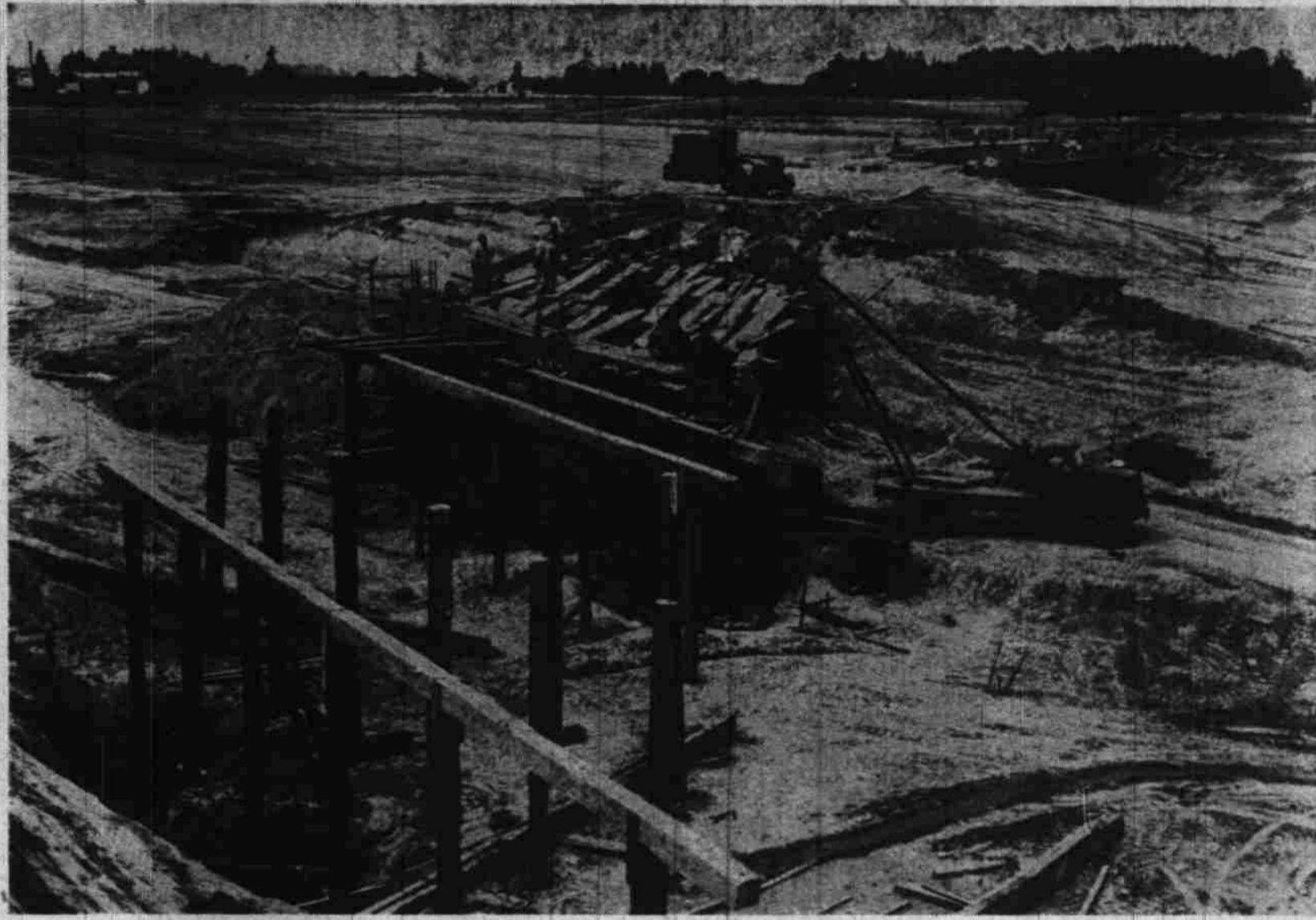
Pile drivers, trucks, earth movers present a busy scene these days near Hayesville on the Pacific Highway just north of Salem, where State Highway Department contract work is in full swing on the big traffic interchange (above) which will link the present Pacific Highway with the new expressway to Portland and bypass east of Salem. (Statesman Photo.)
