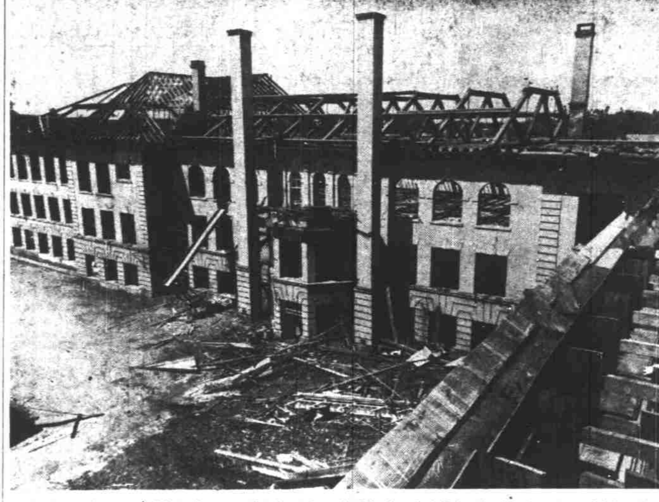
With the roof gone and interior completely stripped, this is what Salem's old downtown high school building looks like now, as wrecking crews continue to raze the structure, making way for new Meier & Frank department store building. Above photo was taken from the roof of the school's gymnasium. (Statesman photo.)
