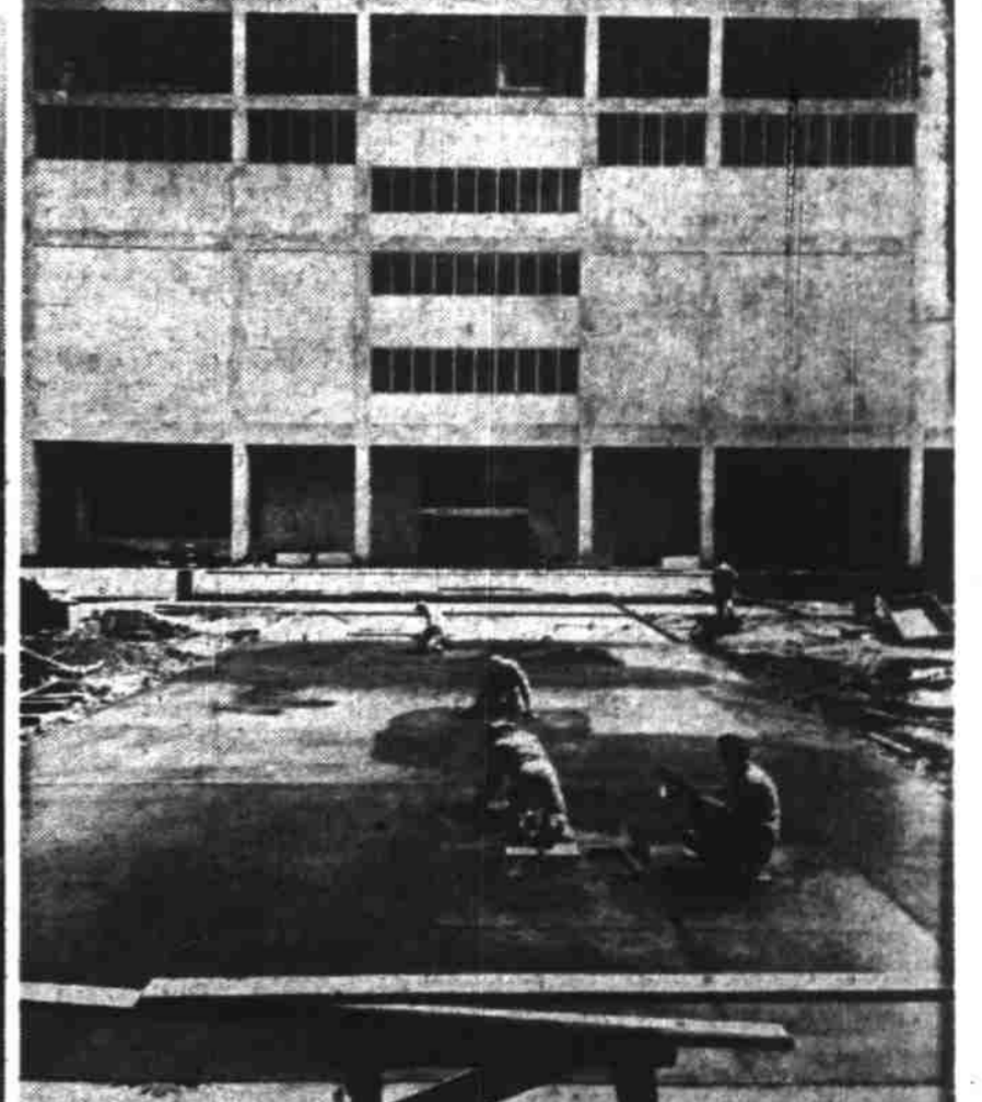
Workmen are shown here putting the finishing touches to the 36-foot walkway, which leads from the High Street sidewalk to the building's main entrance. Grounds on both sides of the walk will be landscaped and planted to lawn. Parking lot is at rear of building.
