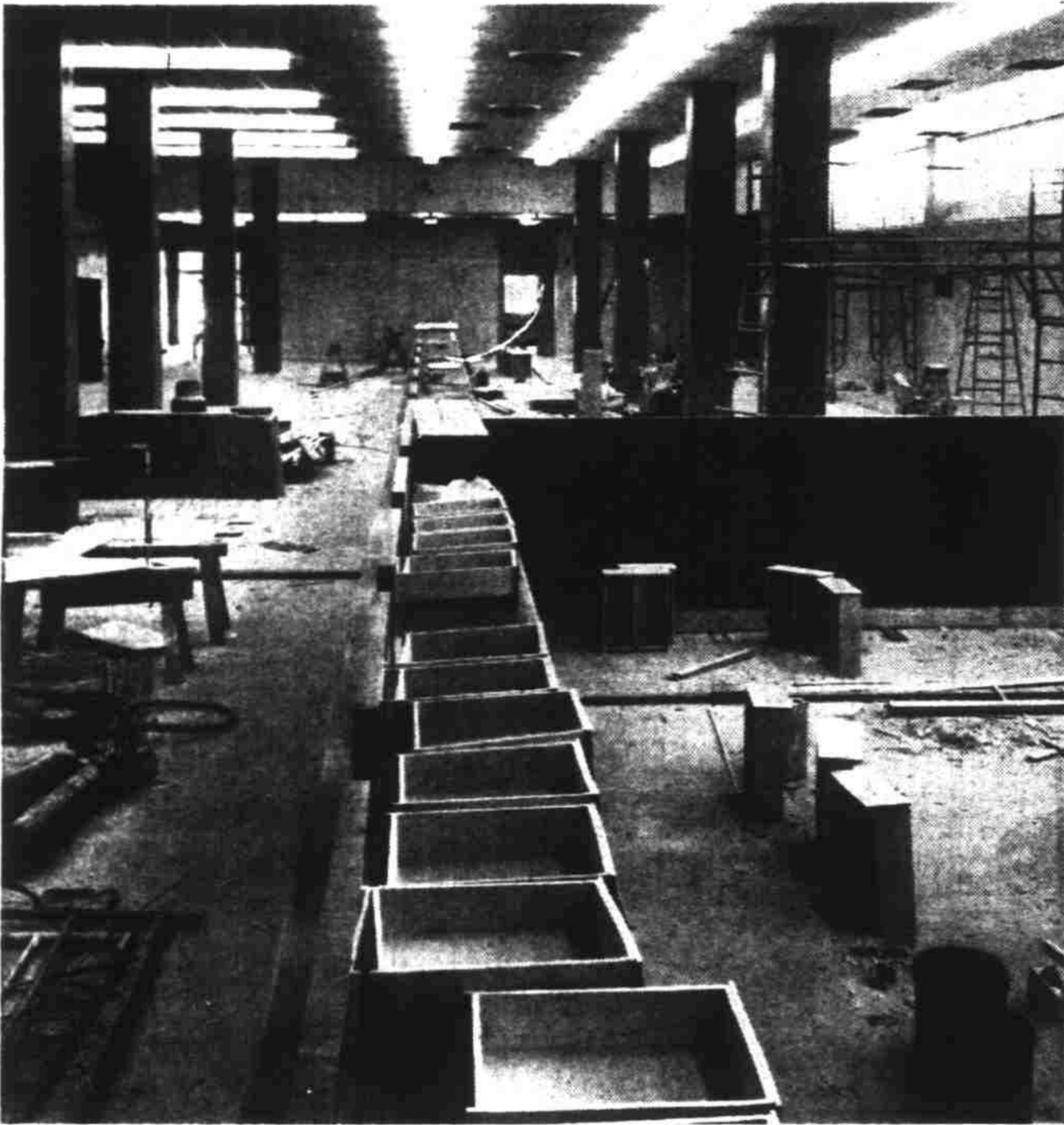
Work yet to be done on the "assembly line" counter on the courthouse main floor is indicated in the photo above. The long counter will serve the county clerk, recorder, tax and other offices. Position of these busy offices on the main floor is for convenience of the public which enters building through nearby main entrance.
