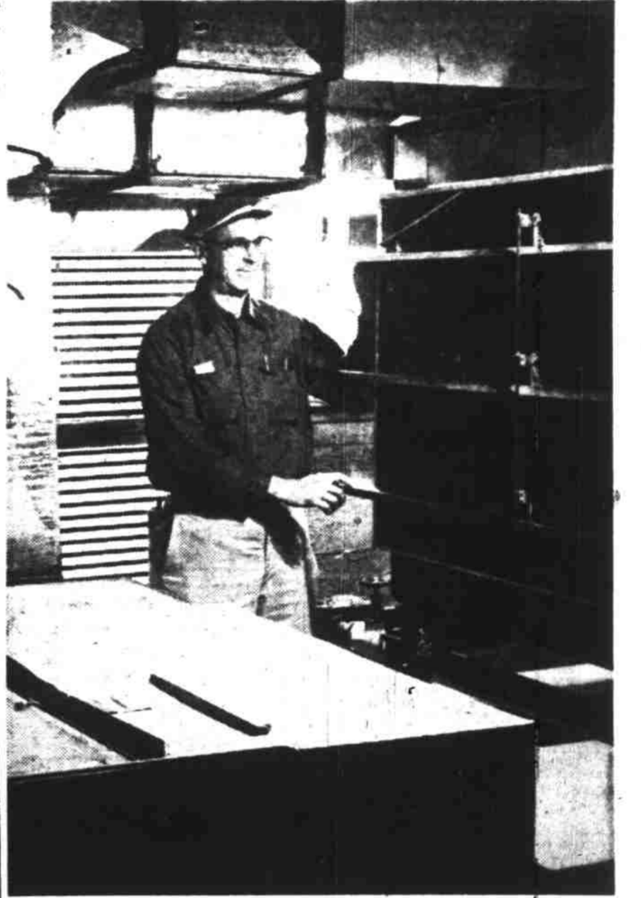
Units supplying air to the third-floor courtrooms are shown in this "penthouse" room (above). W. (Dinty) Moore, mechanic for the Johnson Service Co., examines an intake unit. Similar rooms of units for servicing the rest of the building are located in other sections of the courthouse.
