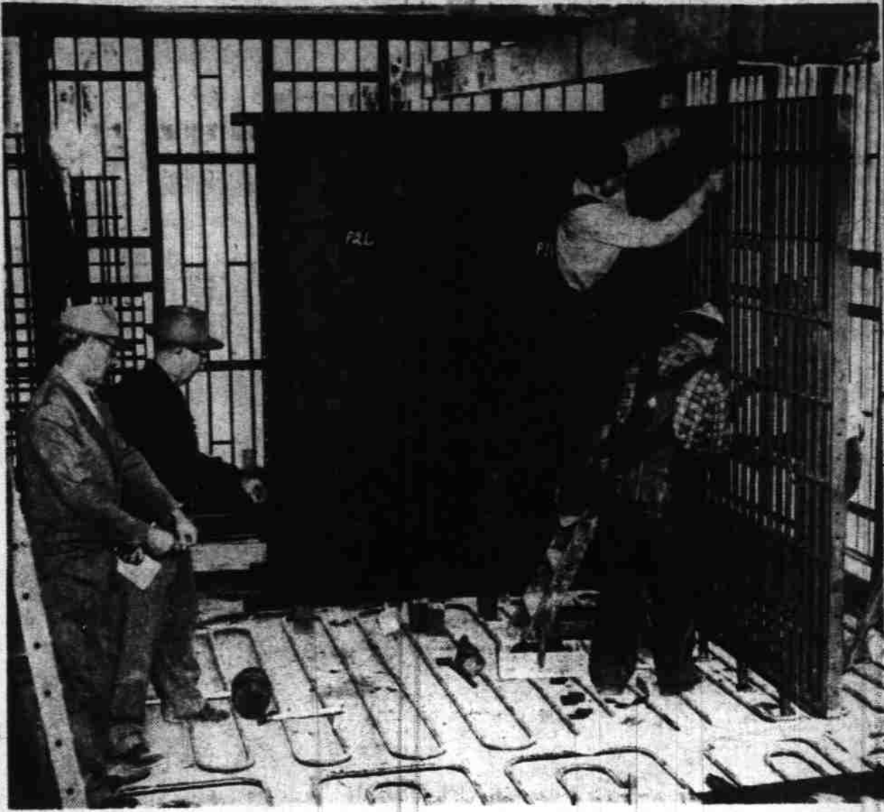
Part of the bars and metal panelling for Marion County's rooftop jail atop the new courthouse is shown above being installed by workmen and supervised by representatives of the Pauly Jail Building Co., St. Louis, Mo., contractors for the job. From left to right are O. A. Hausman, superintendent; Ted Tysdal, foreman; C. L. Nicholson and Fred Clark. In the foreground is shown piping which will be used to heat the jail and after equipment is installed a concrete floor will be poured. In the background is the detention sash which girds the building's top floor. (Statesman photo.) (Story on page 5, sec. 2)
