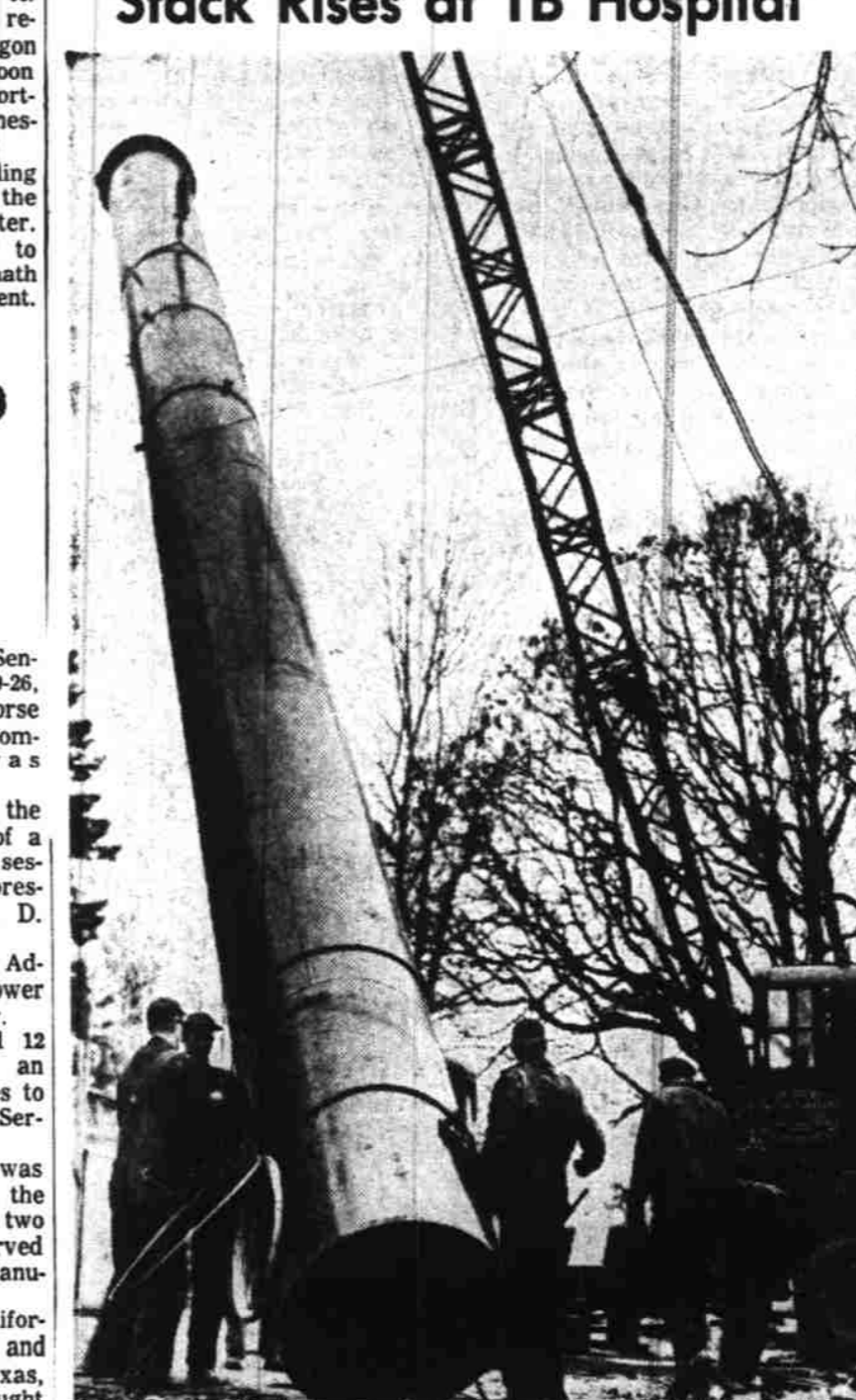
A 72-foot steel smoke stack, shown above, was lifted into place Wednesday over the central heating plant at the Oregon State Tuberculosis Hospital. Weighing 7 tons and 42 inches in diameter, the stack will take care of a 250 horsepower boiler expected to go into operation about Feb. 1. The new boiler will provide heat for a new dormitory and the two new floors of the hospital unit, David T. McKeown, business manager, said. (Statesman photo.)
