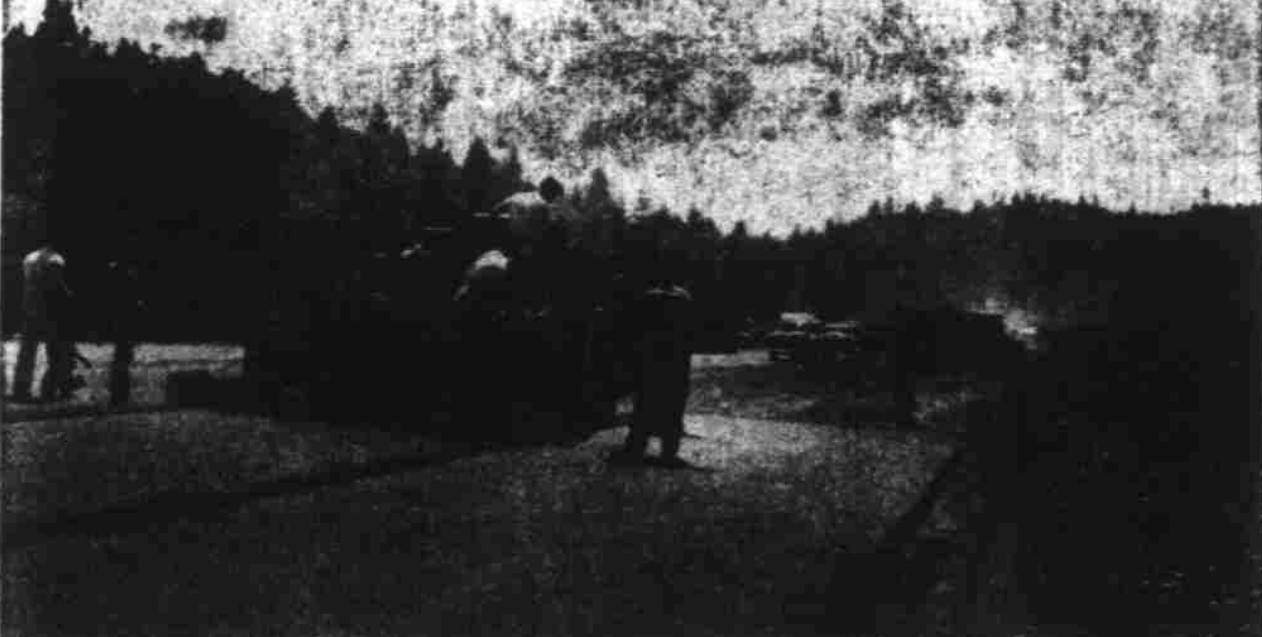
Above, in 1926, they "spread the hot stuff" the hard way on Highway 99E. Below, and later they "laid it along" evenly and easily—more machines, fewer men; four times the progress. (State Highway Commission Photos).
