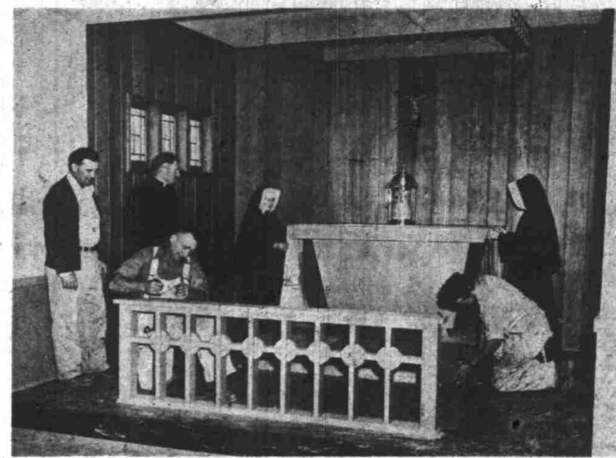
Workmen hurry to finish the chapel in the new Sister's Convent of the St. Vincent de Paul Catholic parish prior to dedication ceremonies today. Left to right: W. E. Schunk, contractor; the Rev. John Reedy, pastor; Les Schroeder and Tom Korn, church members donating labor; Sister Superior Margaret Jane and Sister Alphonsus Mary. (Story also on page 5)
