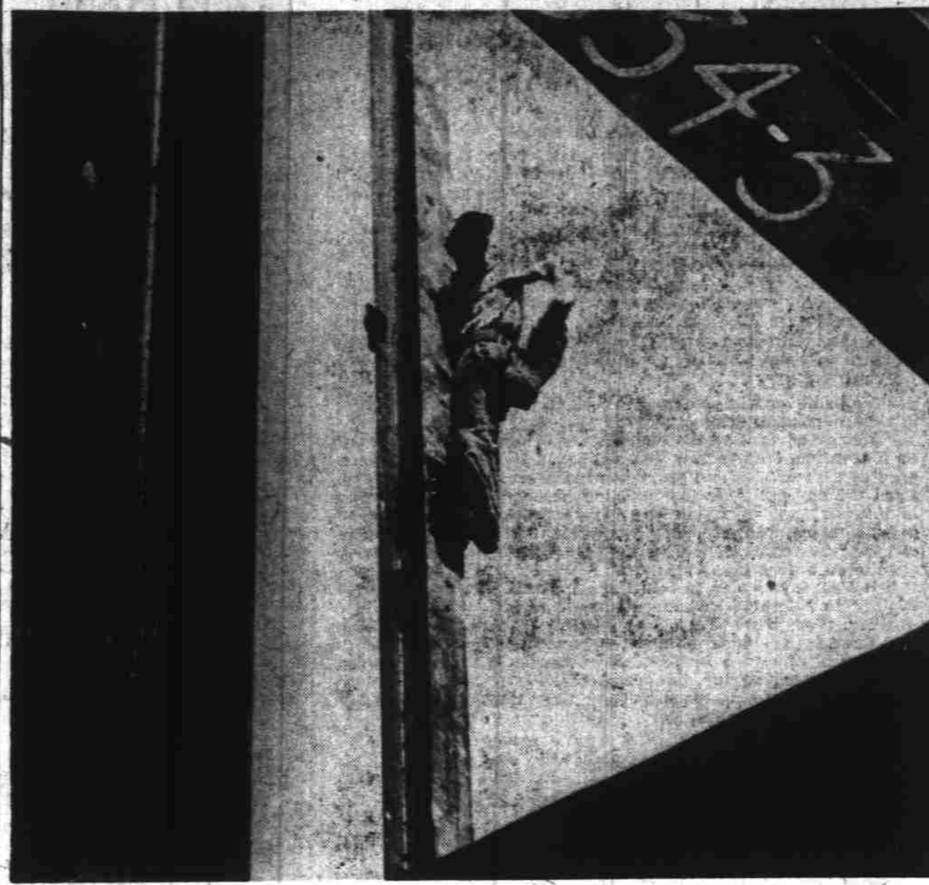
Sidewalk superintendents have been having a field day this week as iron workers perform circus-like feats of daring while erecting the steel skeleton to the new courthouse building. Shown above framed between three steel girders—one of which weighs nearly six tons—is Ted Mackmore, Portland iron worker. Mackmore is standing on a six inch steel brace and hanging on to the girder—100 feet above the ground—with his right hand. (Statesman photo.)
