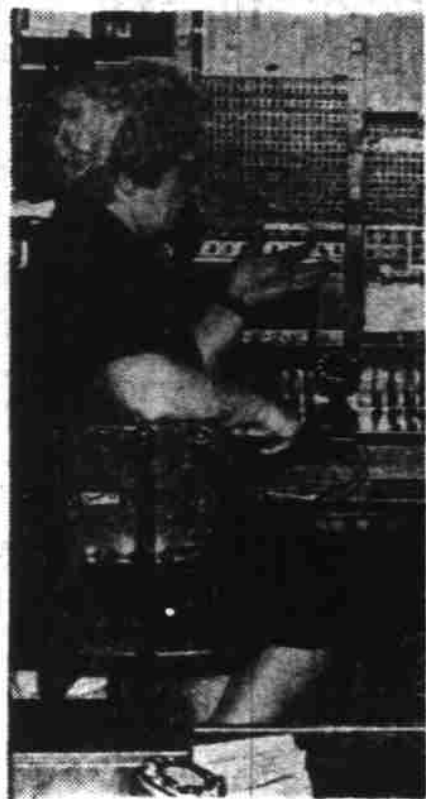
SILVERTON—Lou Hoaland, who had been with the Interurban Telephone Company as an operator for 33 years, is shown here (left picture) making the last "plug in" Saturday night just before the system shifted from central to a dial one. Lowell E. Brown Sr., (right), president of the family-owned company, snips 154 wires to set into motion the $200,000 dial system. Mrs. F. L. Brown, his mother, whose husband started the business in 1905, and Lowell E. Brown Jr., now an employe of the company, are also pictured. (Farm Photo for The Statesman.) (Story on Page 3.)
