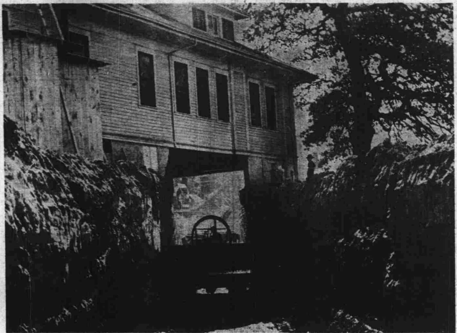
Excavation for the new Salem General Hospital is advancing right under the eye—and offices—of the contractor, as evidenced by this photo. Coming toward the camera is a tractor and earthmover driven by Frank James and operating in the tunnel that will connect the new and present buildings. The picture is looking south-east, with the present hospital in the background. The undercut building is the former nurses' home, now used as offices by the hospital and contractor, Ross B. Hammond Co. of Portland. Most of the excavation has been completed on the $750,000 first-wing project.
