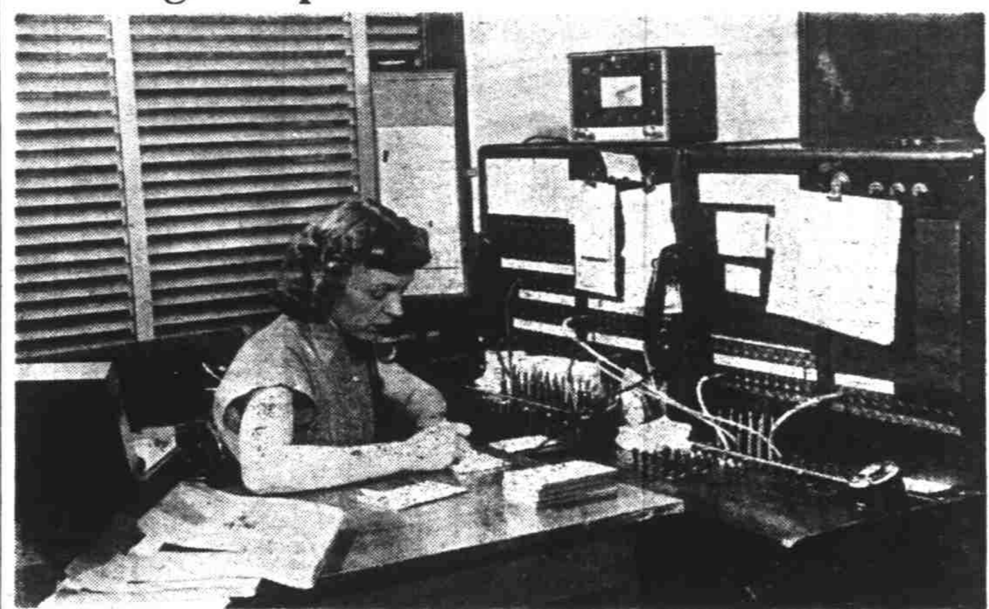
Mrs. Vince Elliott is shown taking a call at the little-known Salem Medical Exchange switchboard. The exchange is operated as a public service by local doctors. Calls, mostly at night, come in over two switchboards from patients seeking to locate doctors.
