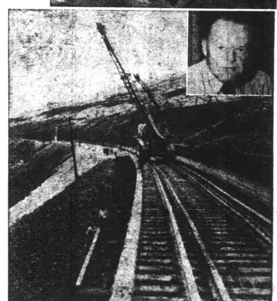
BIG LIFT FOR THE GANDY DANCER. "Caterpillar" Diesel D6 tractor with Hyster Hystaway walks the rails, handles heavy materials for bridge repair at Maupin, Oregon. The Hystaway is a separate attachment for the "Caterpillar" tractor and is readily adaptable as a backhoe, clamshell, dragline or shovel. Inset: Mr. N. S. Westergard, Road Master of S. P. & S. Railroad, where unit is shown in action.
