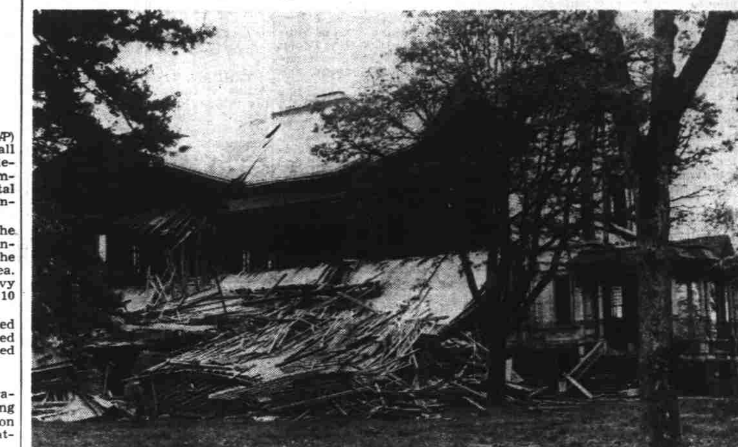
Old Washington school's familiar outline is now gone as wrecking crews work at speeded tempo to remove the building. The familiar landmark will be razed and excavation for a new Safeway store will be completed in about three weeks. Demolition is being done by the Gaylord Construction Co. of Portland. (Statesman photo).
