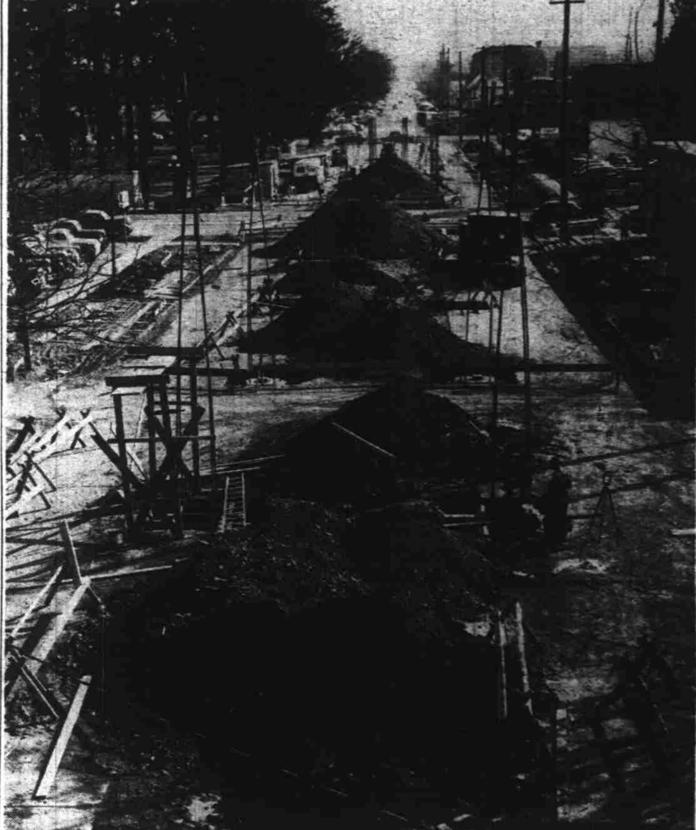
Motorists will see this view of Marion square, upper left, and the area along Marion street from the bridge now under construction across the Willamette river. Mounds of dirt indicate where supports for the long overhead bridge approach are now being constructed. Nearest street above is Front street and at end of construction is Commercial street where the bridge approach will start. (Statesman photo.)
