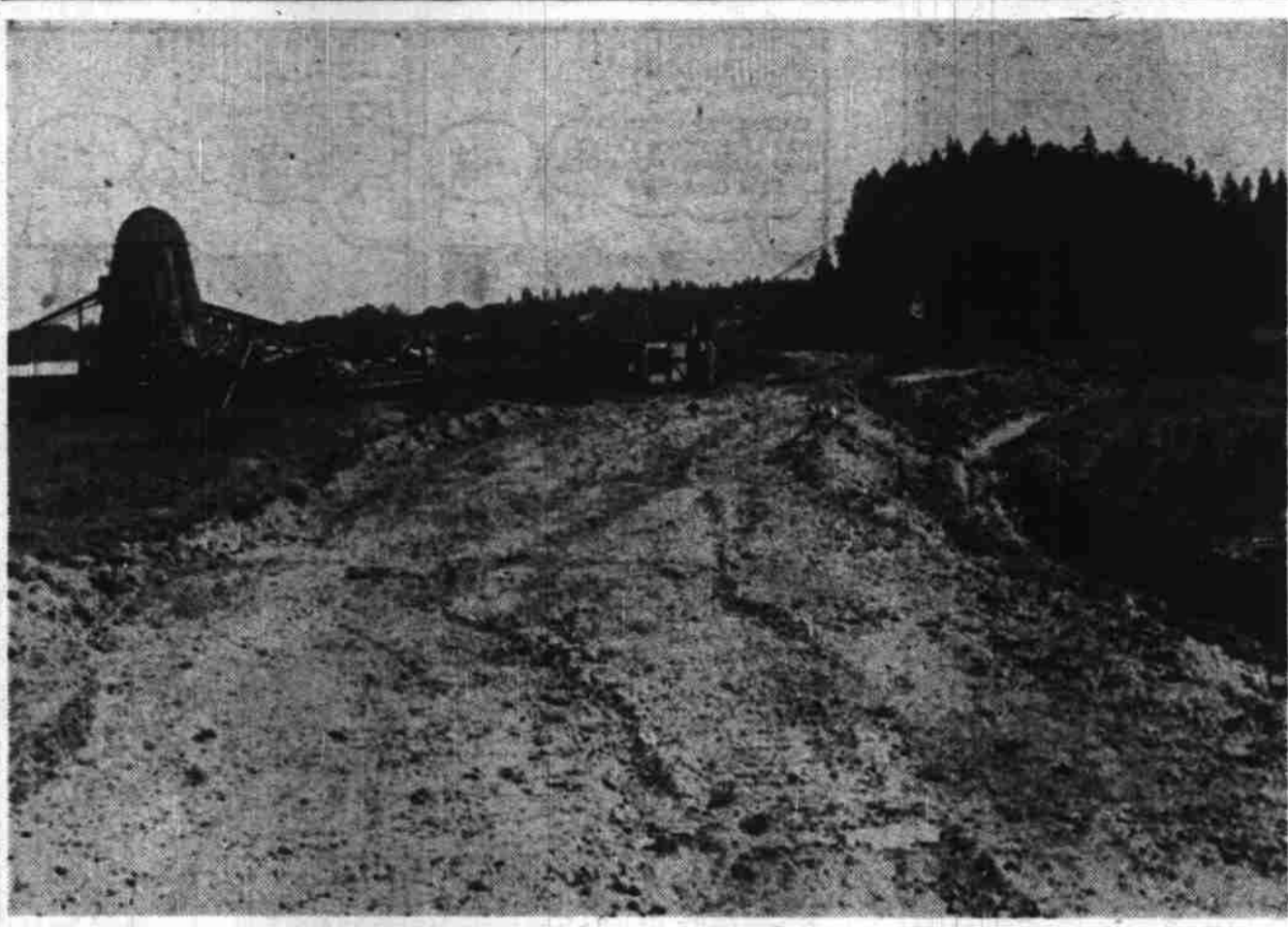
Workers this week have started filling operations to realign the Salem Silverton highway between Brush Creek and Silverton. The new route will run south of the present road, eliminating several sharp curves and providing a wider roadbed. The work is being supervised by the state highway department. (Statesman photo.)
