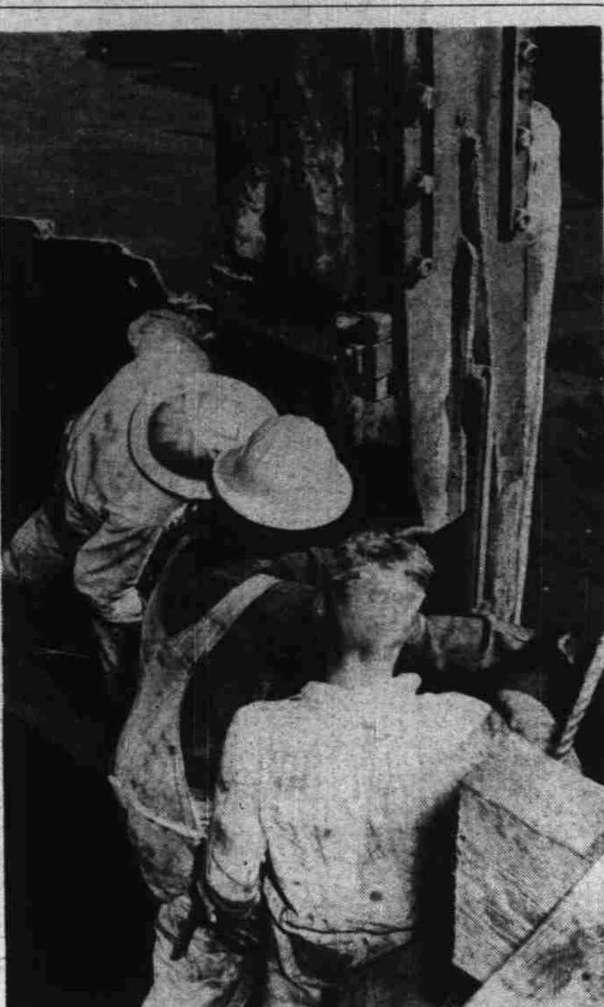
Hoffman company crewmen wrestle huge steam jack-hammer as it drives walls of steel box deep into mud bottom on west side of Willamette river at Salem. When box is completed in river, water is pumped out and pier formations set on river bottom.
