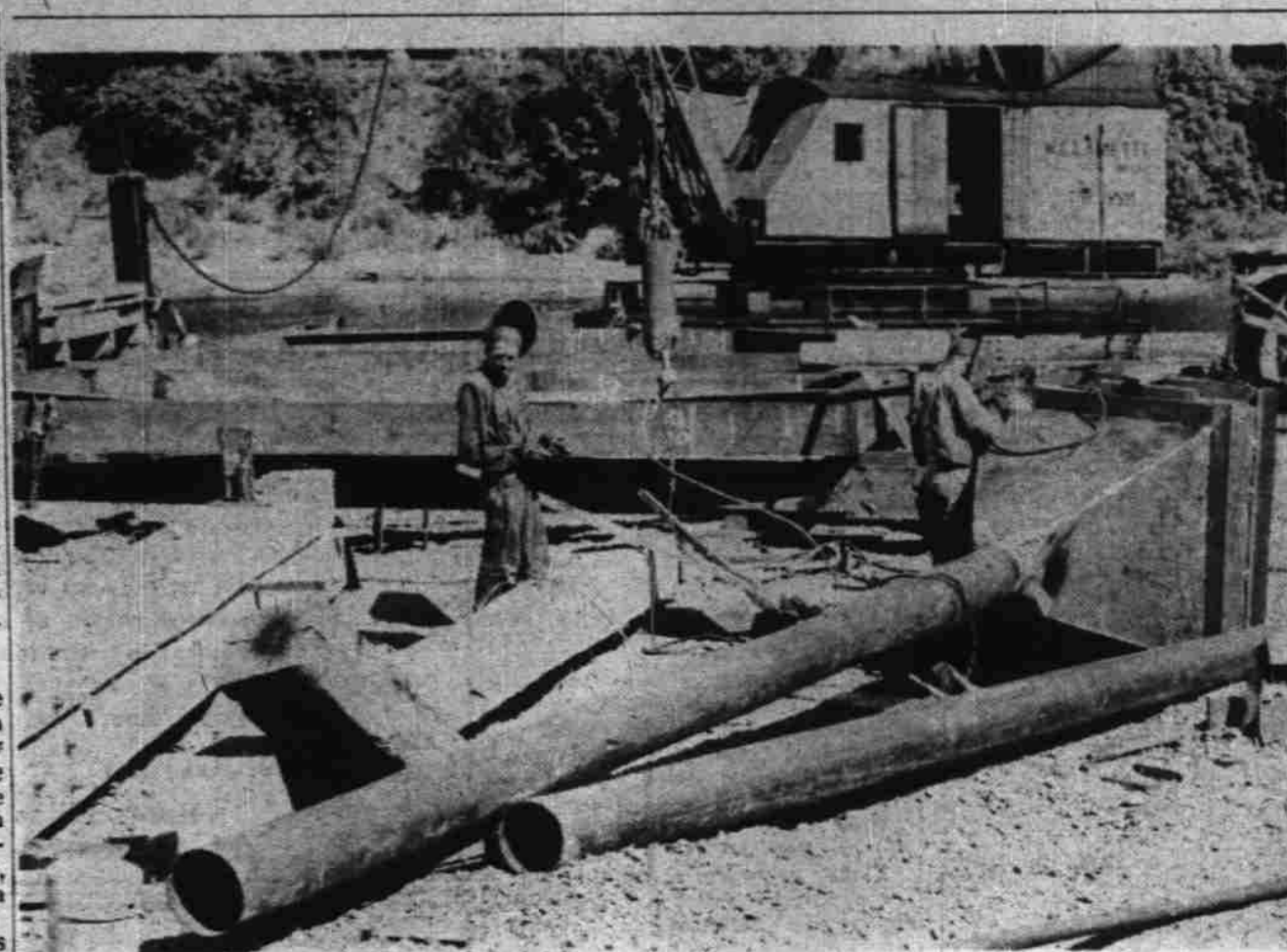
Workmen weld together huge hoppers into which cement for piers will be poured at Salem bridge site. Long pipes go down through water with ends resting on bottom. Concrete is pushed down to form initial cement "sealer" base under water on which piers will be built.
