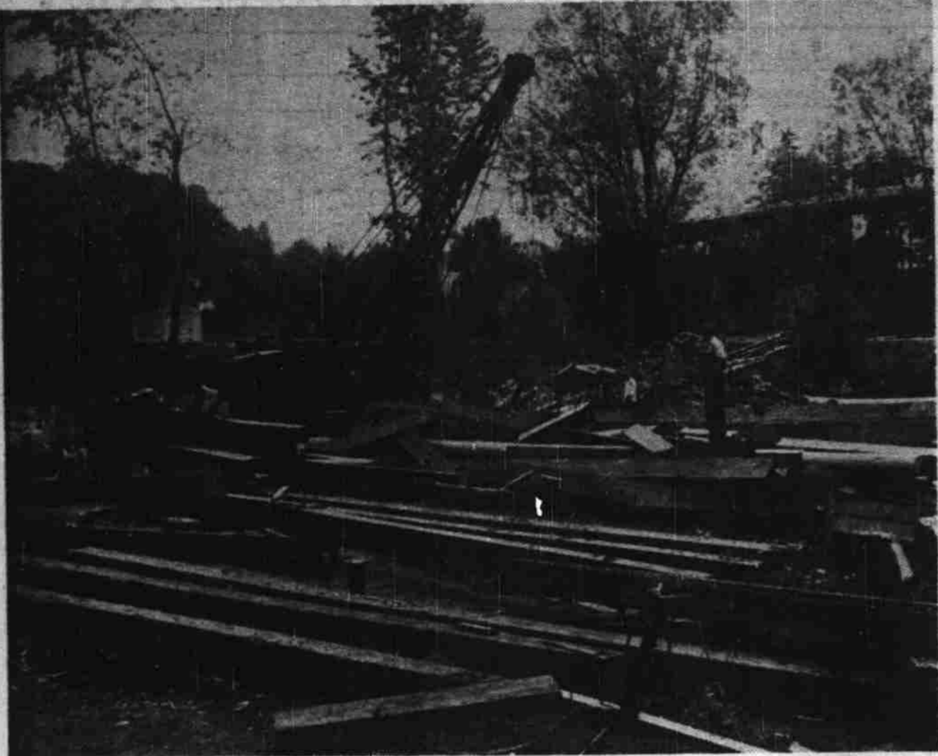
Considerable equipment and materials already have arrived on the west bank of the Willamette river, as pictured above, where work has begun on the new highway bridge, a block north and parallel to the Center street bridge. (Story and photo also on page 1). (Statesman photo).
