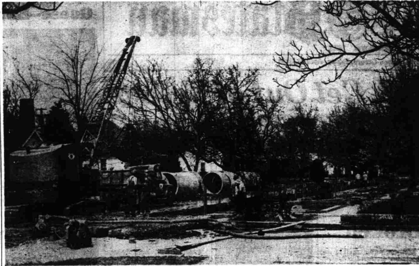
Salem's two mile interceptor sewer line will be completed late this afternoon as the last huge section of concrete pipe is put into place. Above is the last section of ditch to be cleaned out by the clamshell shovel at Belmont and N. 5th streets. The section is on N. 5th between Belmont and Market streets. The sewer line is 60 inches in inside diameter at its beginning at Union street and increases to 72 inches at the future site of the sewage disposal plant on the Willamette river at the north city limits, according to assistant city engineer J. F. Fitzpatrick. Started last August, the pipe was laid by the M. C. Werner contractors of Eugene at a cost of $217,000, Fitzpatrick states. The pipe, manufactured by the city of Salem, cost $150,000. Streets along which the sewer line follows will be paved, some paving having already started Thursday, and other paving due to start today. (Photo by Don Hill, Statesman staff photographer.)
