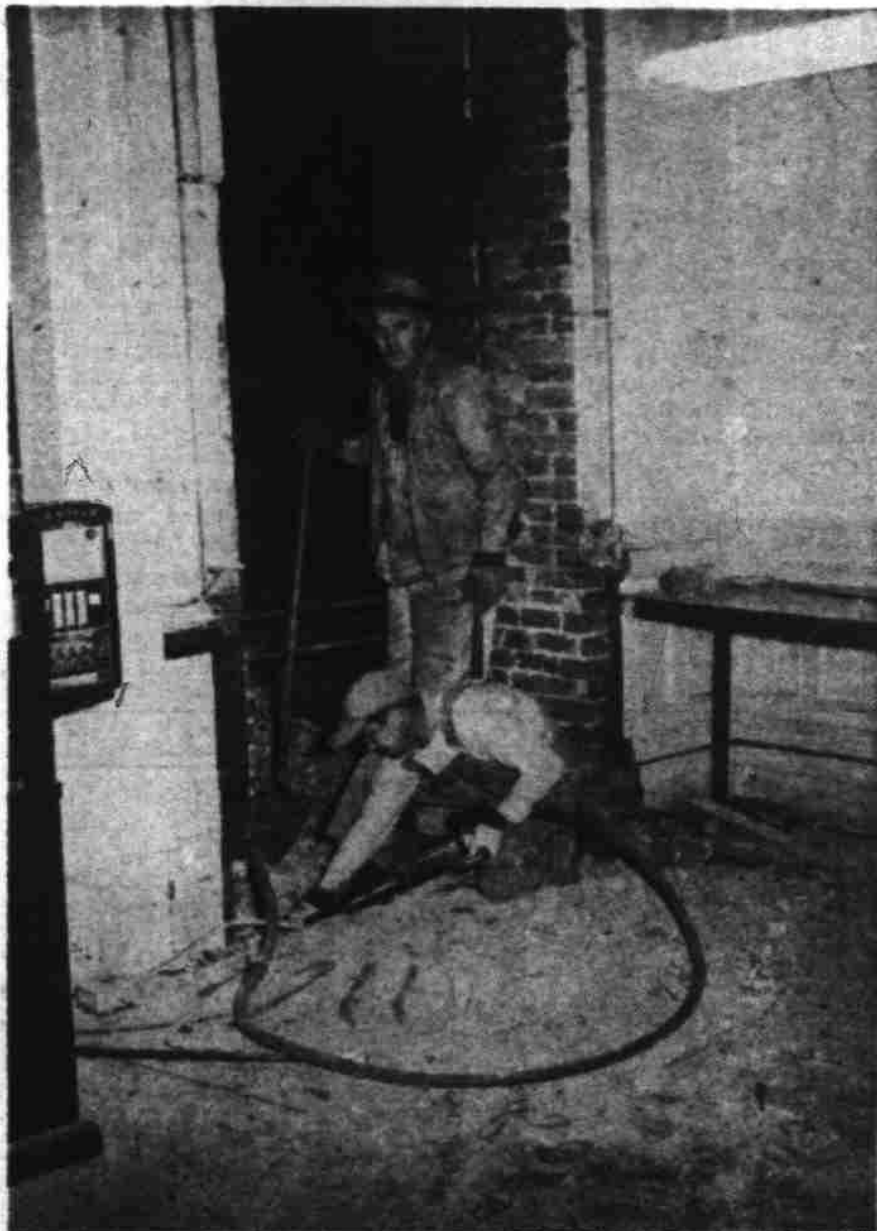
Workmen are preparing a temporary entrance to Salem police headquarters as work begins on a $7,000 addition at the south side of the city hall front steps. Above, working in a cloud of dust, are Paul Hamrick, Salem route 6, with air drill; and A. C. Thomas, Salem route 7, standing. Other photo shows the best known swinging doors in Salem, the present entrance to the police department through which many a solid citizen has marched to pay his dues in the overtime parking club. These will be torn out for the new addition. (Statesman photos.)
